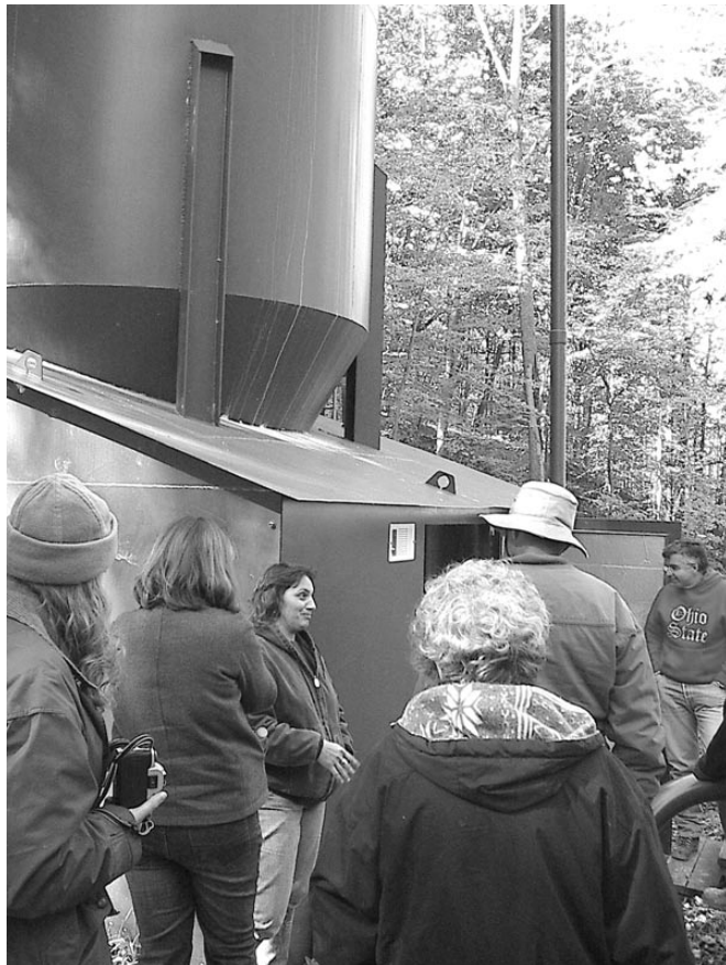
Rebecca shows off the new doser, which is located at the entrance of the Essex Mine off State Route 216.
